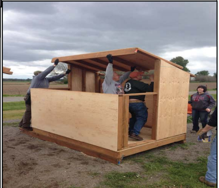
Daren Hauswald, Bob Taylor, Dan Hafenbrack and Ryan Weston sliding the roof into place.
