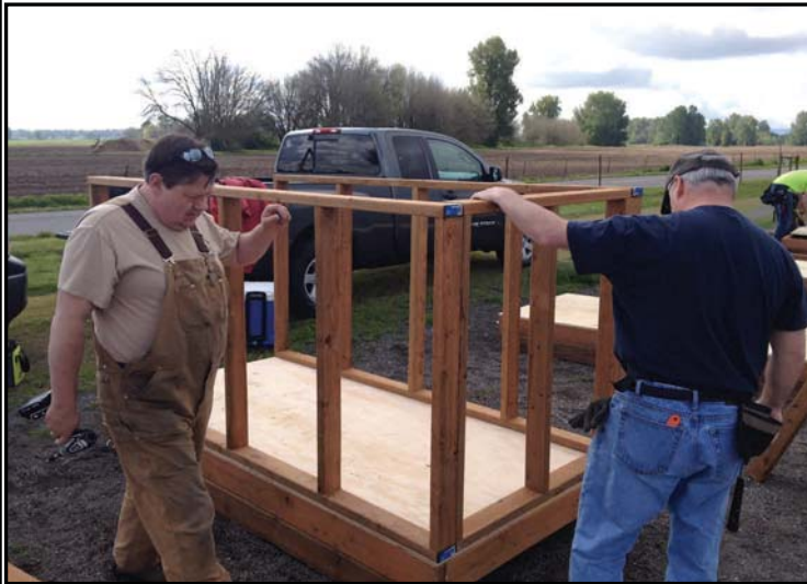
Rick Scott and Ted Blade framing the blind for use at the Shillapoo State Wildlife Area.
