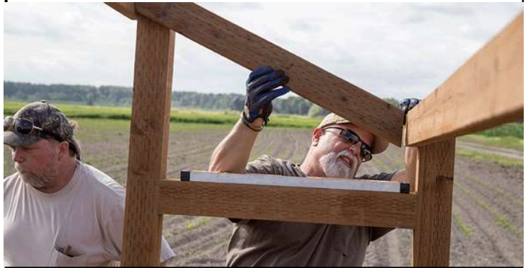
Project organizers Rick Erickson left and Rick Spring attach the roof framing.
