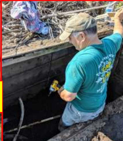
Rodney Vandersypen led the group who removed the old beaver lodge from the pit blind. The beaver had burrowed through the side of the blind and underneath the floor. The entire lodge had to be removed stick by stick, then the floor removed, dug out, replaced and repaired. The seat had to be raised so this blind may not be comfortable for some of our taller members, but it will hunt well.
